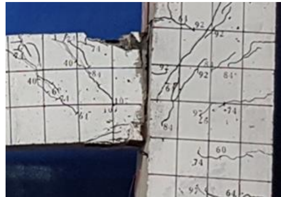
d) PC2 试件边节点裂
