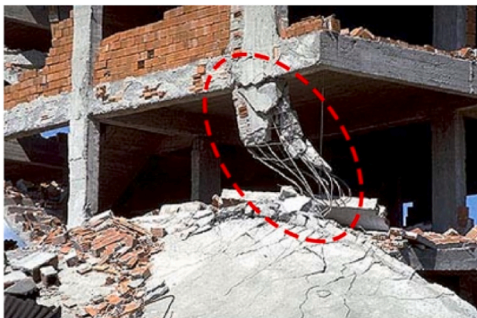
Fig. 1. Failed RC column due to impact of an adjacent building [14].
