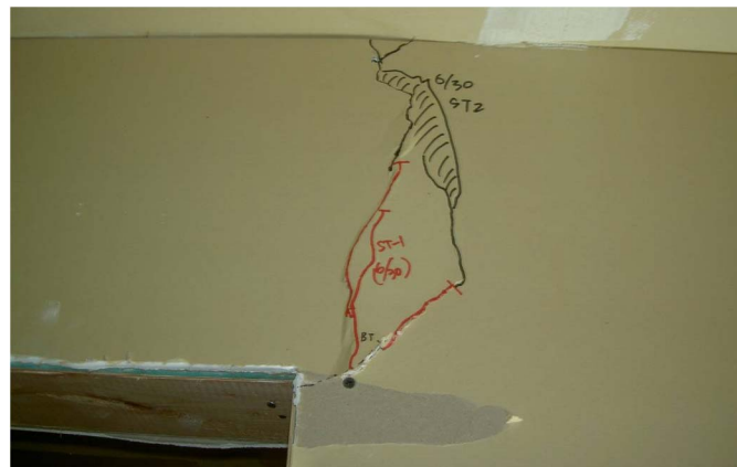
Fig. 9. Crack on Wall D1, Story 4 (over door opening) after Seismic Test 2
