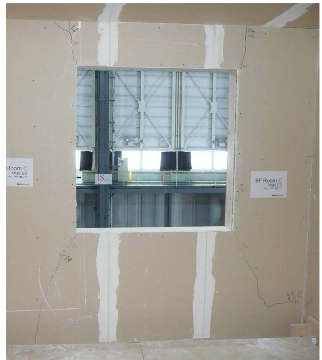
Fig. 20. Story 6, Wall E2; cracks develop all the way through panel for all corners after Seismic Test 5
