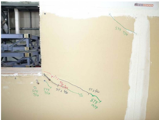
Fig. 17. Wall E1; cracks did not extend all the way to the panel edge after Seismic Test 5
