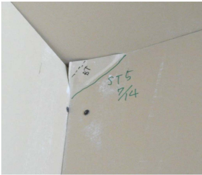
Fig. 21. Crushing of corners also seen at Story 6, Wall E5 after seismic test
