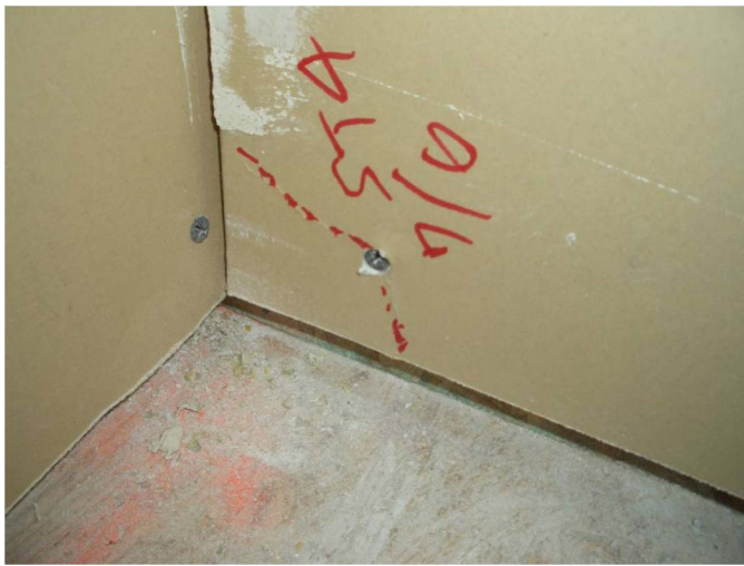
Fig. 12. New crack on Wall D1, Story 3 (corner crushing) after Seismic Test 4
