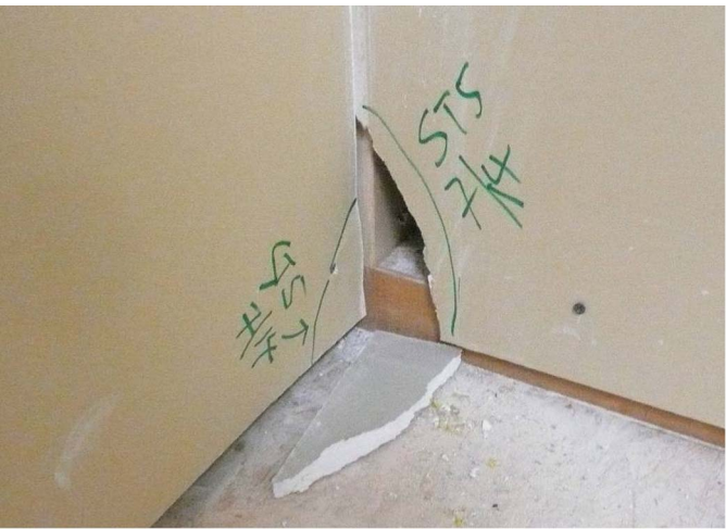
Fig. 15. Crack on Wall D2, Story 6 (corner crushing) after Seismic Test 5
