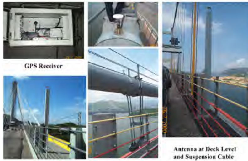
Figure 23. Typical GPS sensory system: GPS rover station at upper deck level and main suspension cables.
