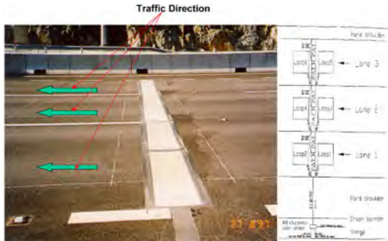
Figure 19. Dynamic weigh-in-motion sensors for Lantau fixed crossing.
