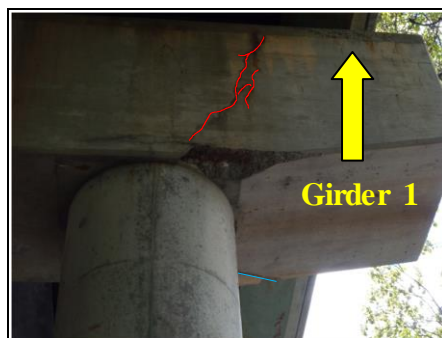
Fig.9. Pier cap crack under girder 1
