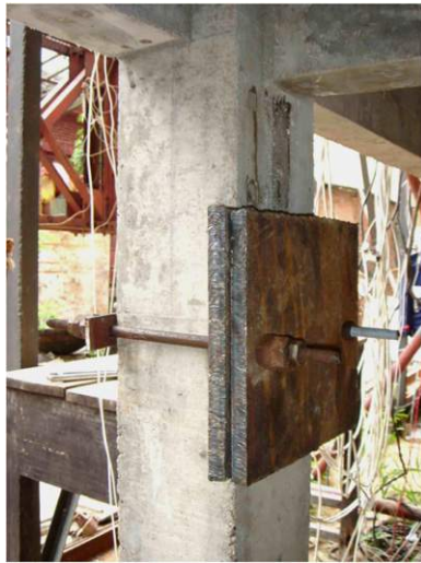
Fig. 8. Additional mass attached to target column.
